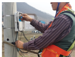
Work Belt on the telephone pole
